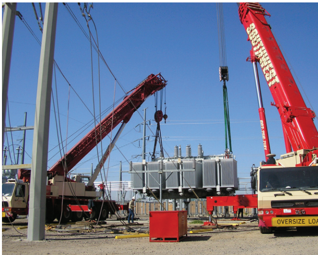
200 ton Electric Transformer
